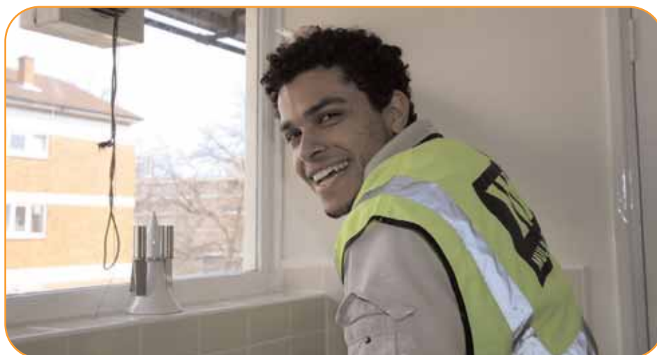
One of the Decent Homes team puts the finishing touches to a kitchen on the Suffolk Estate, Queensbridge. This was one of 184 kitchens installed as part of Hackney's Decent Homes programme in April and May this year.
